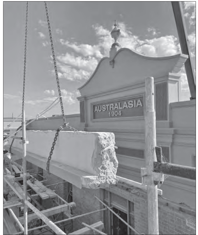
Removing the reinforced suspended concrete parapet that had been installed in the 1950s from the restored façade of Eden's historic Hotel Australasia
