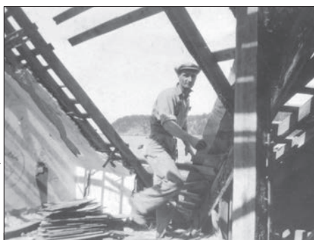
Above: Removing Welsh slate from the roof at the front of the Seahorse Inn.
